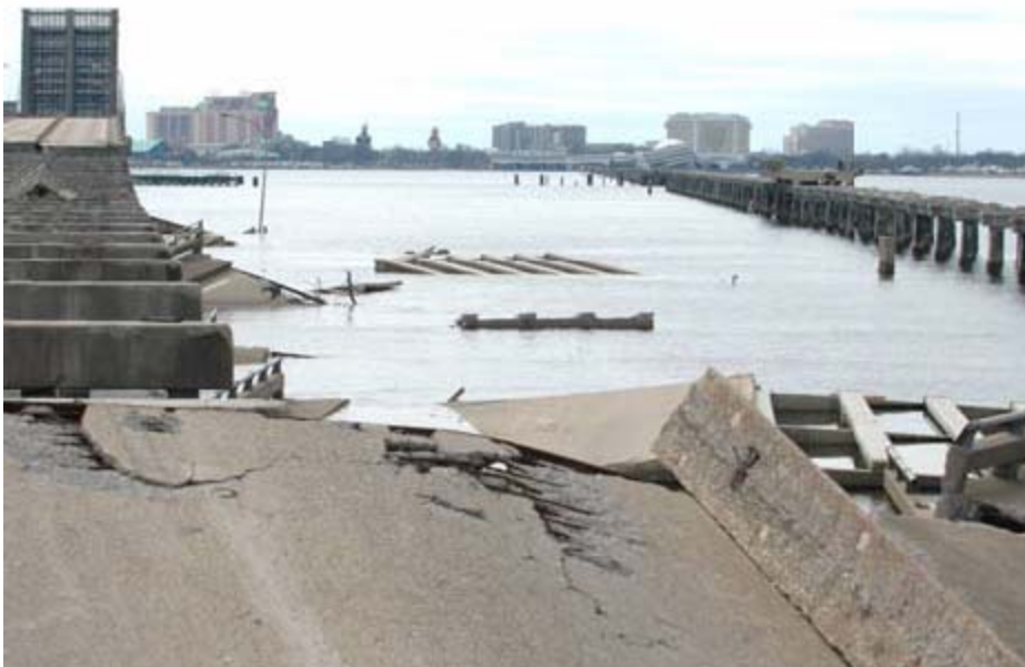
Figure 2 - U.S. 90 bridge over Biloxi Bay, MS, after Hurricane Katrina in 2005. Bridge deck spans were moved off the substructure and several spans were flipped (center of photo).
