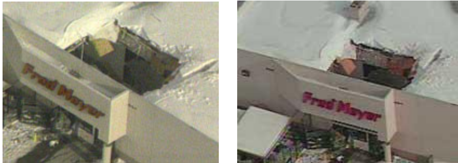
Figure 3 – Partial collapse of Fred Meyer store roof in Portland, OR, January 10, 2004. (photo from KGW.com)
